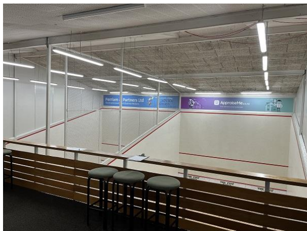
New court lighting
