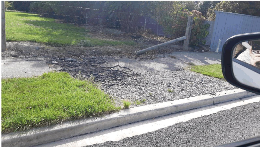
Pembroke Street - Footpath and Road damage typical of these streets (SLIDE 15 and 16)
