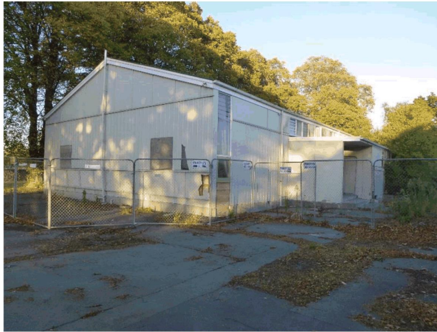
Former Burwood Community Hall – after the 2011 event and now demolished (SLIDE 19)
