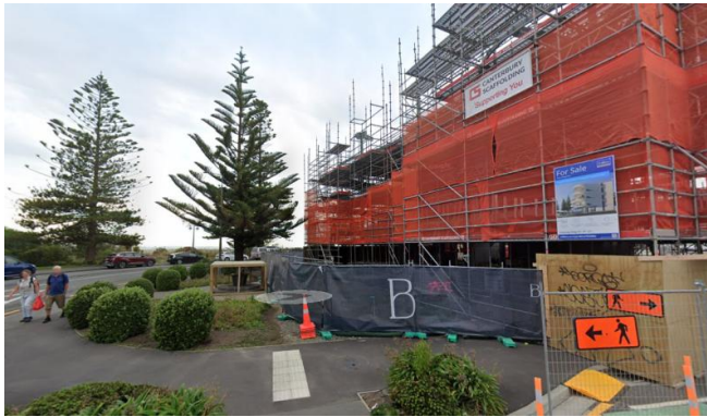
Above – Google street view of 2 Esplanade (April 2025), showing Beachside scaffolding occupying the site.
