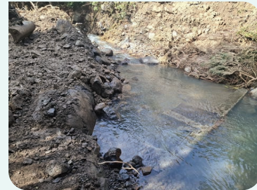
Little River - Police Creek water supply intake during February 2026 storm event.
