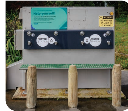
Chlorine free water station on Keyes Road, New Brighton.
