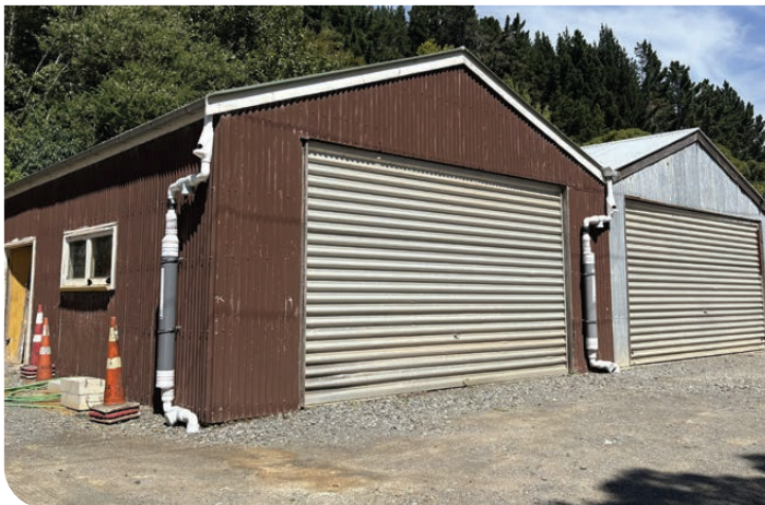
Storminator installed in Akaroa Wastewater Treatment Plant.
