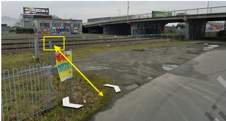
Rectangle – Lockable gate for access to insert ramp Arrow – constructed safe pathway being installed
