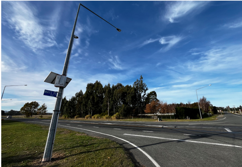
Example of SMART Assessment Camera in Operation
