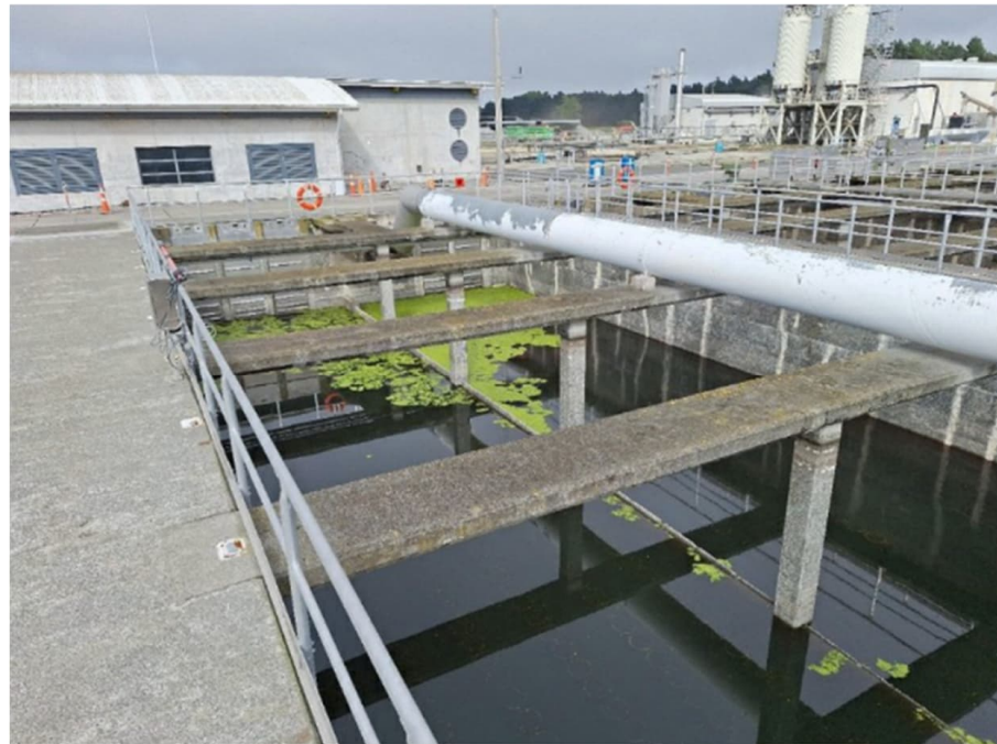
Lane which has been out of service for a couple of months
