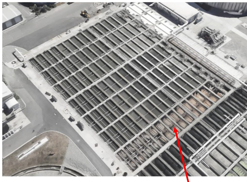
Aerial image showing the 7 PST's, with the Eastern tank drained
