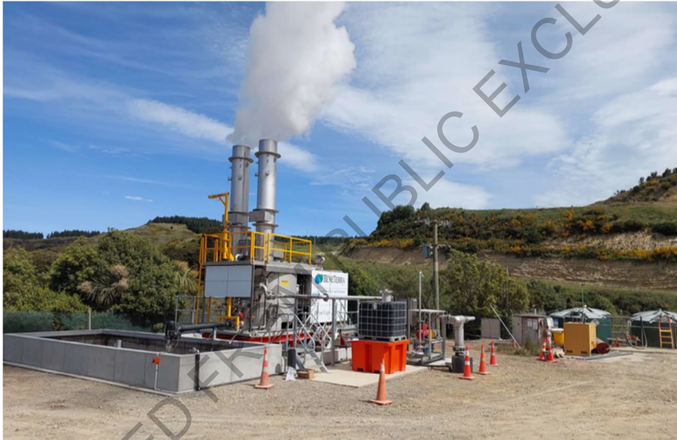
The new BeneVap landfill gas powered leachate treatment plant – reduces road transport emissions by treating on site using and destroying methane from landfill gas (visible plume is steam)
