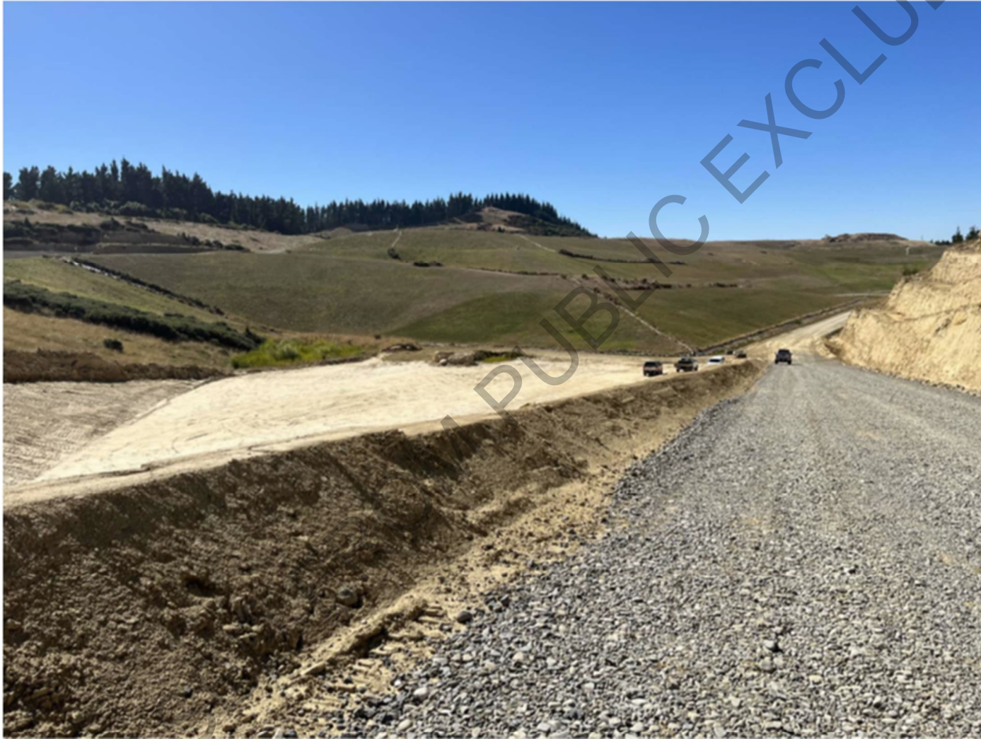
The new cell Phase 5A under construction looking toward the current landfill
