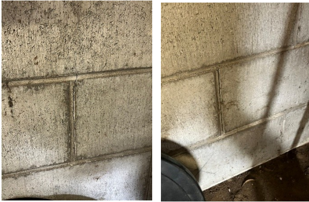
Figure 5: Photo showing examples of minor cracks
