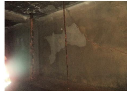
Figure 25 Large area of lining lost from wall.
