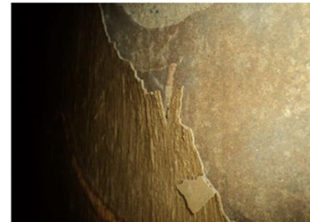
Figure 27 Lining cementitious base layer with friable to layer over.
