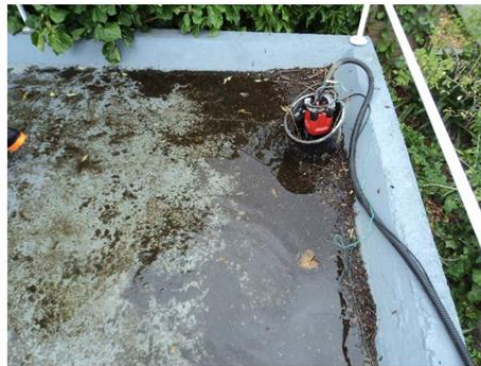
Figure 20 Ponding in south-west corner.
