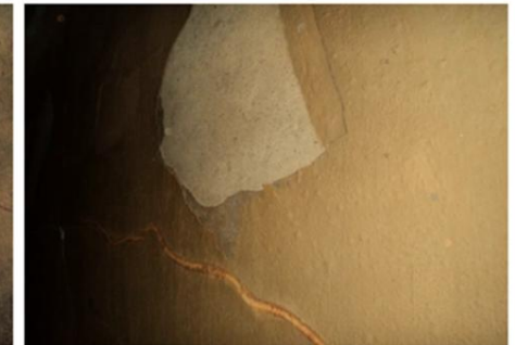
Figure 26 Large area of lining lost from wall and repaired crack.
