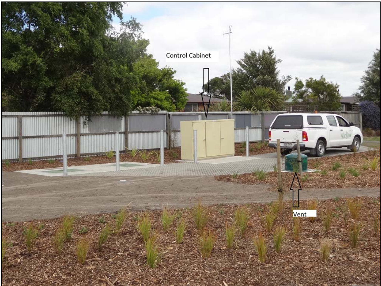
Example of a similar Pump Station to that proposed at McFarlane Park. Note: The vent is a Green Dome O
